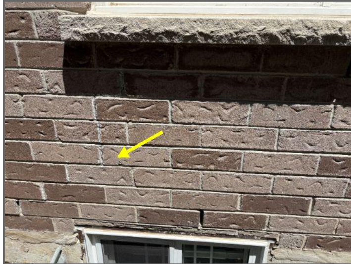
Minor wall crack noted.
