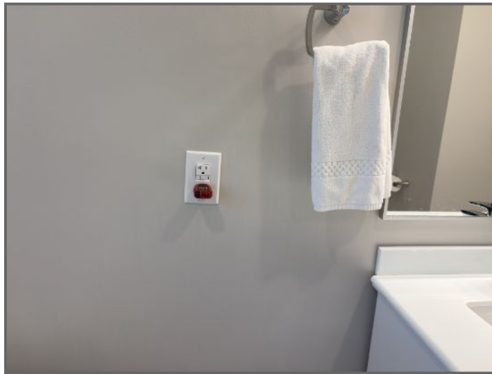
Primary bathroom outlet doesn't operated.
