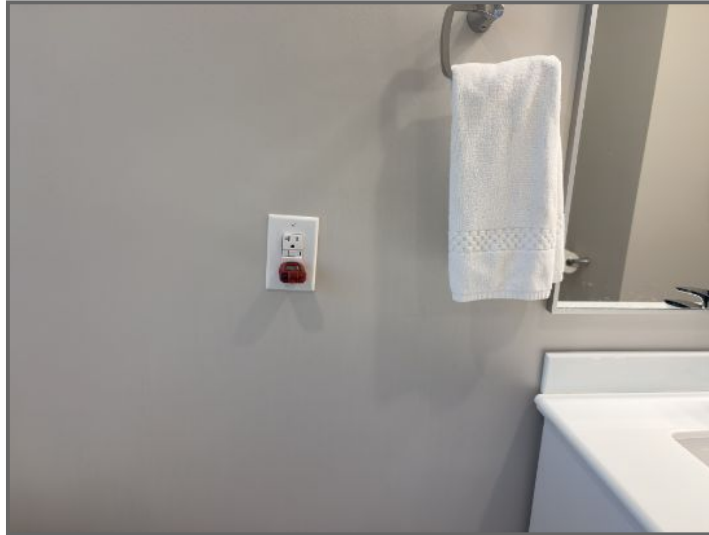
Primary bathroom outlet doesn't operate.
