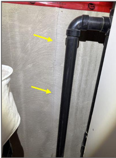
Minor crack noted.
